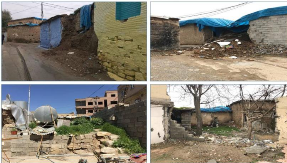
Figure 12: some views shows the demolished or inconvenience situations of the residential units (by researchers).
